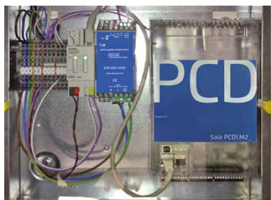
Connection to an existing EIB/KNX installation providing conference rooms with a web connection
